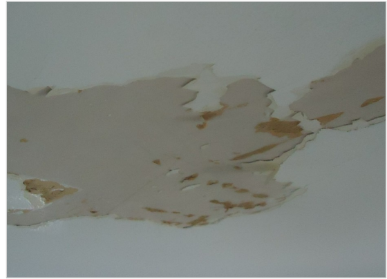
Second-floor bedroom ceiling, directly below the slope shown above. Staining and paint failure consistent with water entering at the damaged courses.
