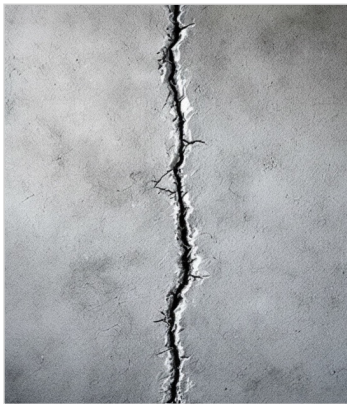
Foundation wall, north elevation. A vertical crack runs the height of the pour, with efflorescence along both edges where water has moved through it.
