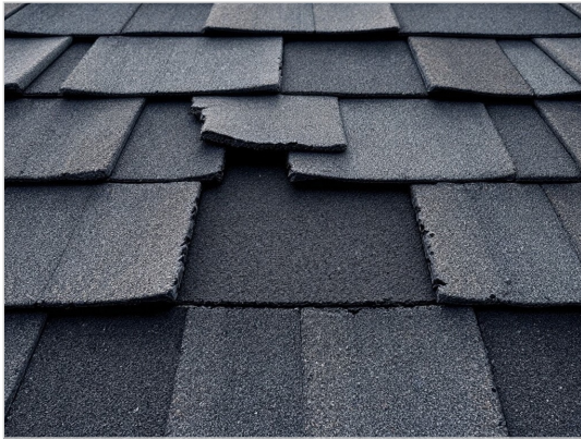
Roof, west slope. Shingle tabs are cracked through and displaced from their courses. The covering is the original 1994 installation. Photographed 14 March 2026.
